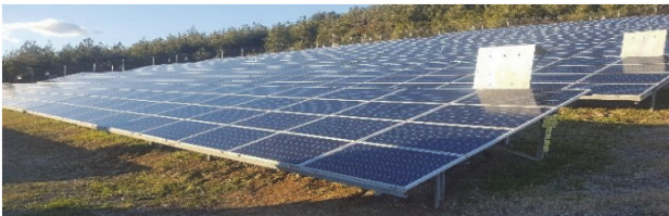
Figure 1 Image of the PV array
