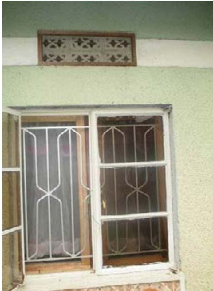
Figure 4. A ventilator and window with screening on one of the demonstration houses.
