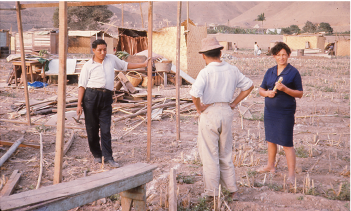
John Turner, Construction of El Ermitaño, Photograph, in Golda-Pongratz, "John F.C. Turner (1927-)"
