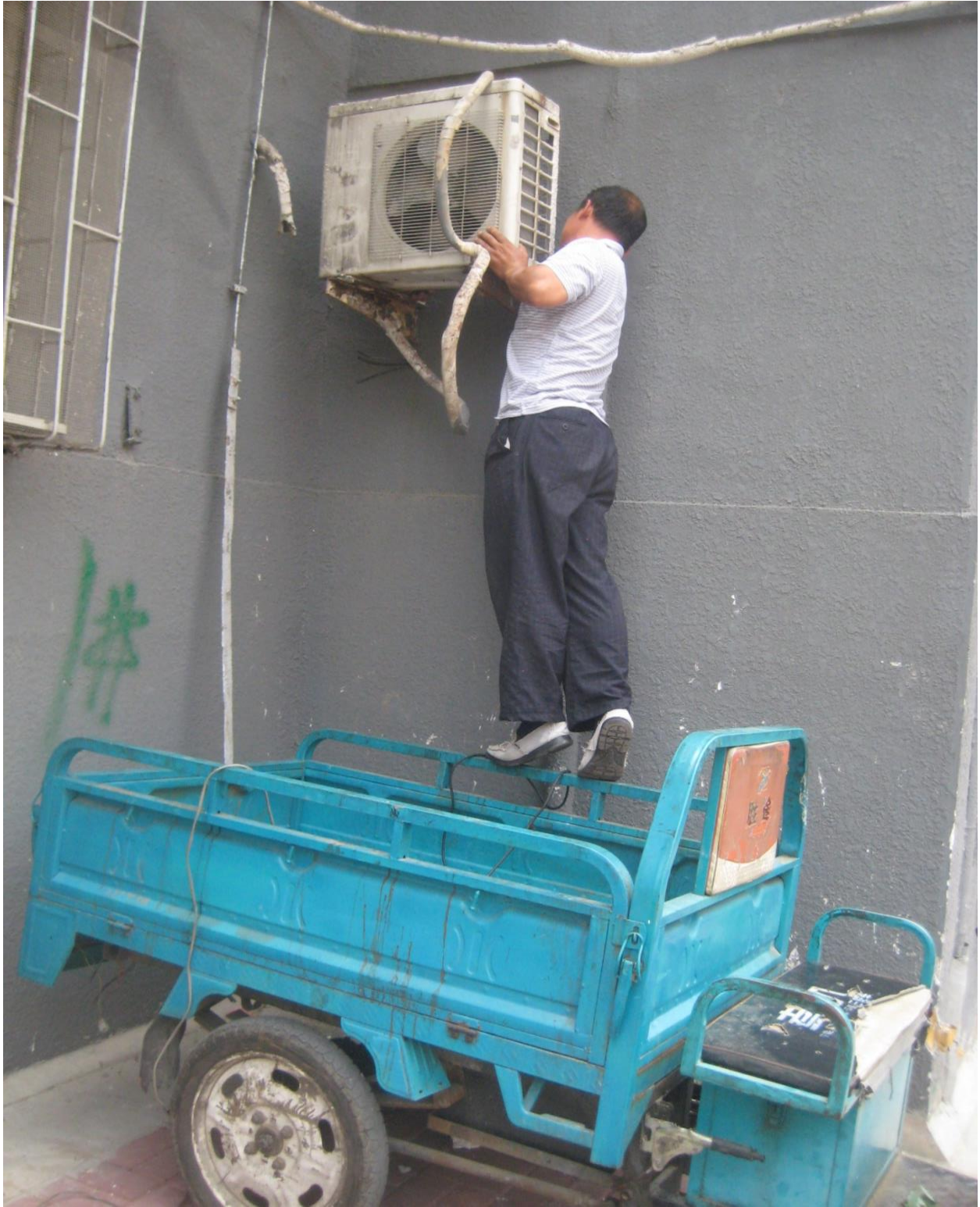
Fig. 3.2 Mr. Ma removing an air conditioner from a building after purchasing the appliance.
