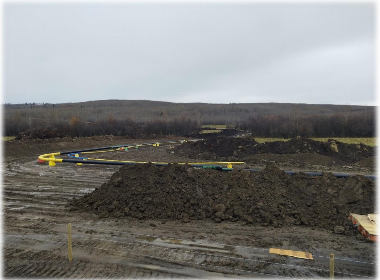
Figure 30 - Construction works of a gas pipeline section in Northeastern BC. Picture taken by Giuseppe Amatulli on October 16 th , 2019.
