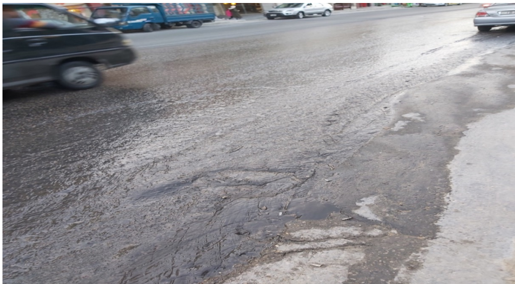
FIGURE 7.12 SEWAGE WATER FLOWING IN ONE OF THE STREETS IN THE EAST SIDE OF AMMAN
