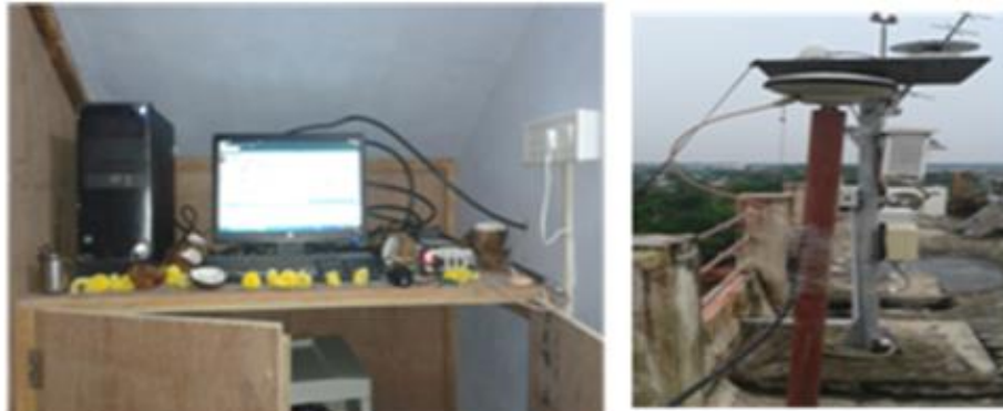
GPS Receiver station at IMD, Machilipatnam (16° 12' N, 81° 08' E), Dual Frequency GPS Receiver and Antenna (Model: GPS Station6 Make: Atel), Installed on 20th September 2014 Sanctioned under DST Project, File No: SR/S4/AS-91/20121
