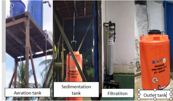
Figure 5. Clean Water Treatment Equipment Pondok Pesantren As – Shiddiqiyah
