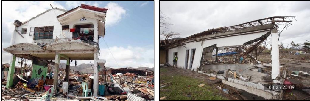
Figure 2: The aftermath of Typhoon Haiyan in the coastal areas of Tacloban City, Leyte: (a) Two-storey residential building with collapse masonry wall at the groundfloor, (Pedrasa, 2013) (b) A bungalow house with collapse exterior wall and damaged roof but RC frame is intact. (Edds, 2014)
