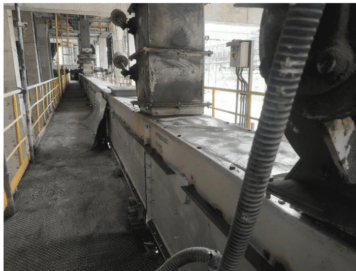
Gambar 2. Mesin Chain Scraper Conveyor
