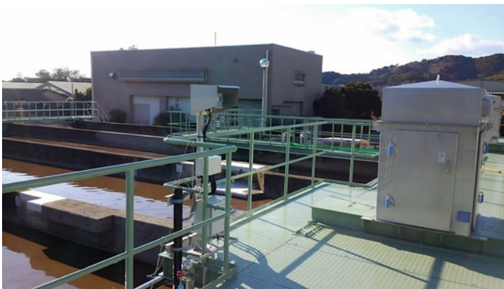
Fig. 11.1 Oxidation ditch at Yasu WWTP, Konan, Japan. (Photo: provided by Maezawa Industries, Inc.)
