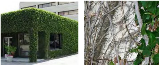
Fig. (4) Ivy attaches to a building using aggressive adhesive suckers or climbing roots that can damage surfaces and enter voids and cracks.
