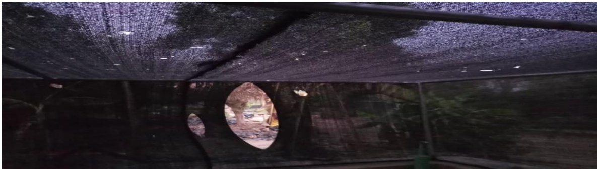
Figure 3: shows a completely damaged cocoa shade net by the forest fire in CRIN nursery.
