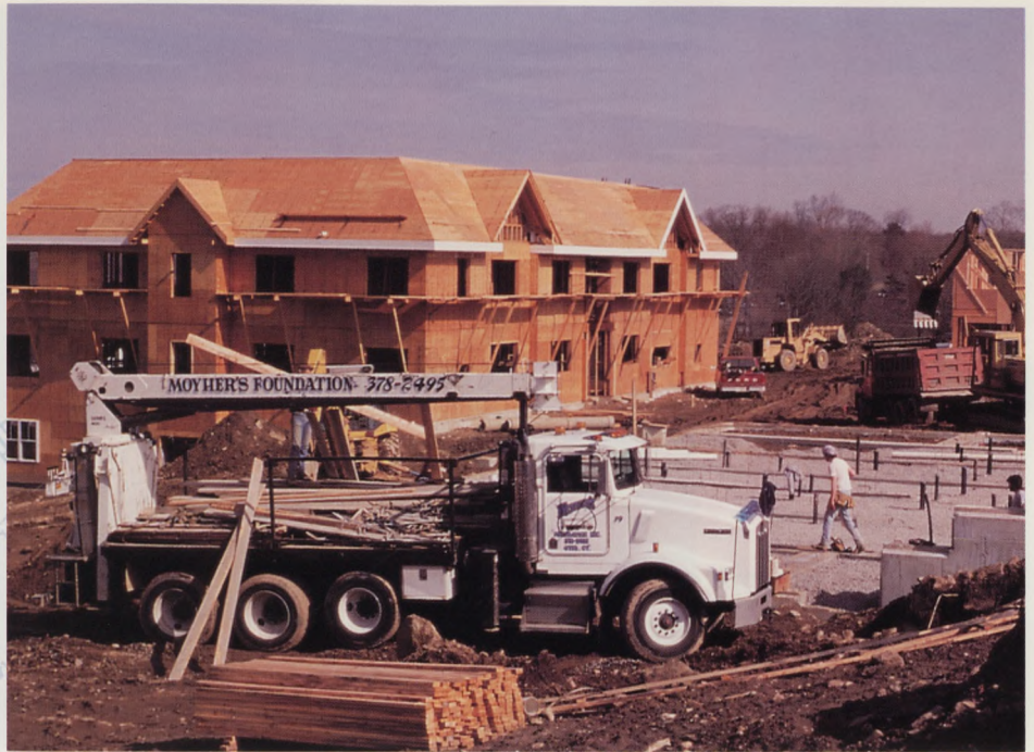
Construction continues on SHU's four new residence halls slated to open in August of this year.
