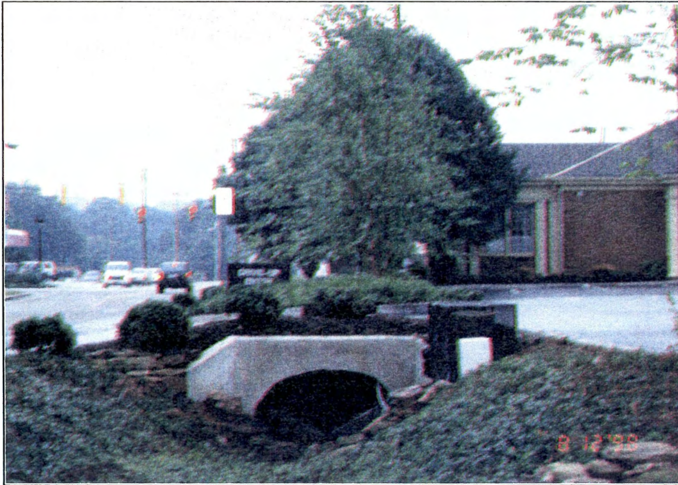
Figure 4.4. Looking downstream at the Church site. Weir is located within a box culvert, which is approximately six feet downstream from the oval pipe opening.
