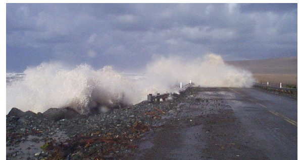
California Highway 1 before realignment with high swells, San Piedras. (Figure source: Caltrans).
