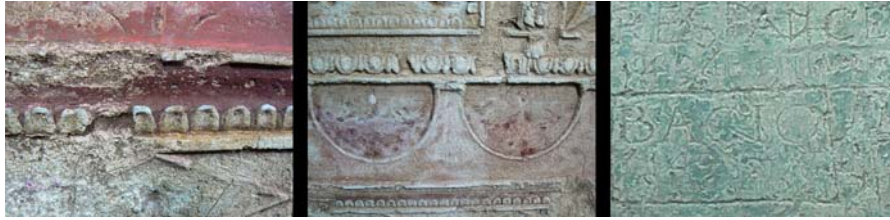
Figure 2. Reference areas characterized by deterioration (left), salt emerged on surface (center) and graffiti (right).
