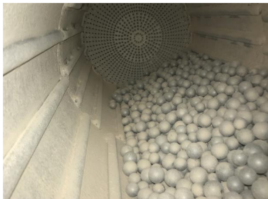
Figure 5-23: Empty mill during pre-trials with air velocities of > 1\text{ m/s} above the ball filling
