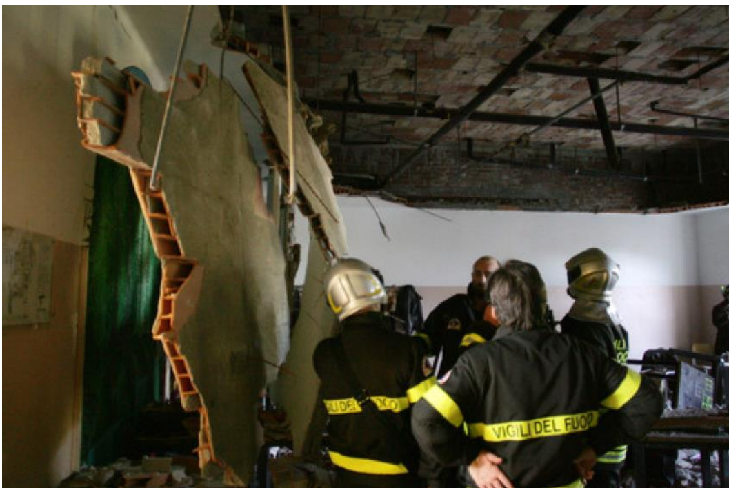
Fig. 25: Illustration of the ceiling collapsed at the Darwin High School in Rivoli, Turin, Italy.
