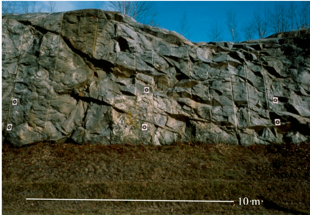
Figure 2. Photograph of a N5E striking roadcut exposure at the study site on I-93 containing NE striking, SE dipping faults included in this study. Note, most of the faults fractures exhibit dark planar surfaces. The rock type is primarily Concord granite (dark gray) with a Lower Rangeley schist block (light grey/white) exposed to the right of center above where the grass meets the bedrock and between the first and fourth drillhole from the left side of the photo. The subvertical lines are drill holes used in blasting the roadcut surface. Targets were used for rectification of photographs on which the geology and fractures were mapped by [16] (sheet 2).
