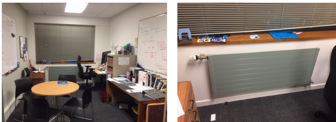
Figure 4. Manually controlled radiator in a typical office.
