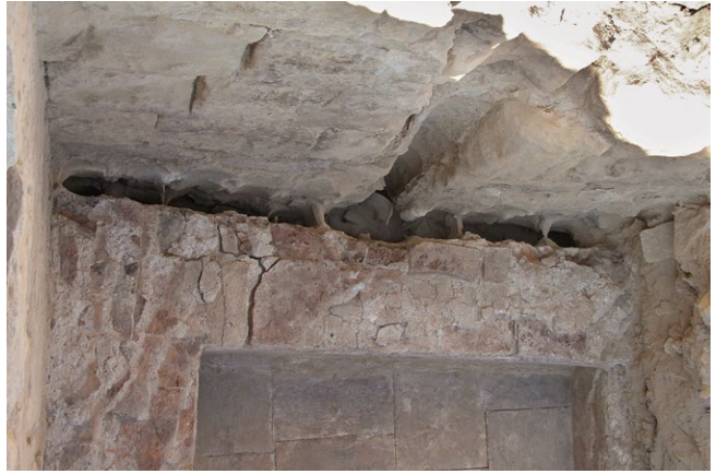
Fig. 38: Elusa (Haluzá), bath complex. Sondage 17, detail of lateral wall, pool enclosure and tubuli in between, looking NE
