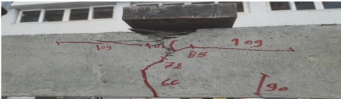
Figure 16: Typical failure modes of normal concrete sleepers at rail seat section: (a) SN-No.4; (b) SN-No.5.
