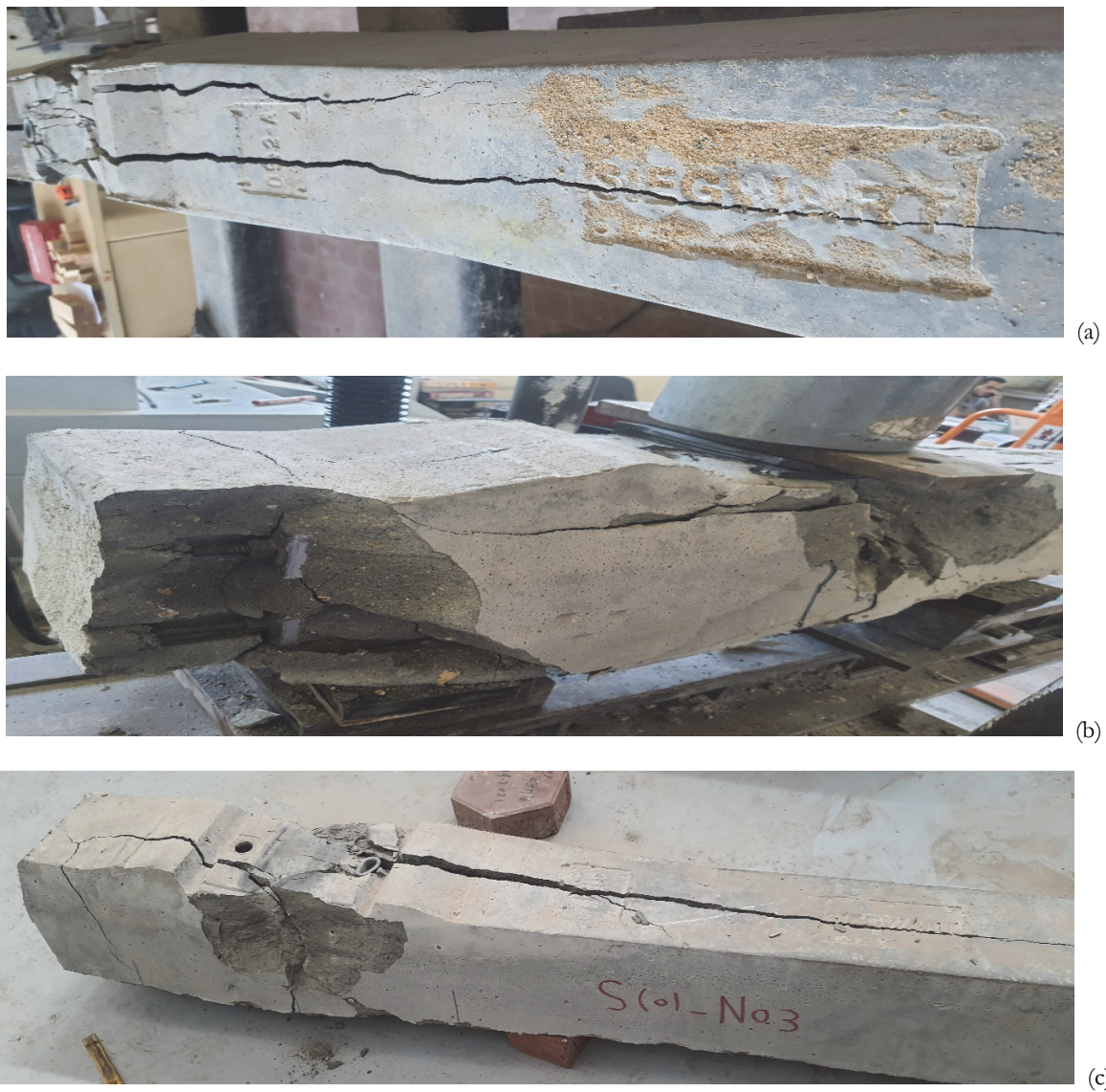
Figure 13: Typical failure modes of UHPC concrete sleepers at rail seat section: (a) S0-No.1; (b) S0-No.2; (c) S0-No.3.
