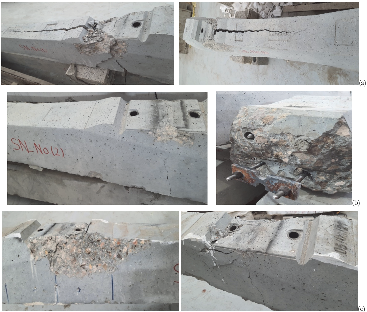
Figure 12: Typical failure modes of normal concrete sleepers at rail seat section: (a) SN-No.1; (b) SN-No.2; (c) SN-No.3.
