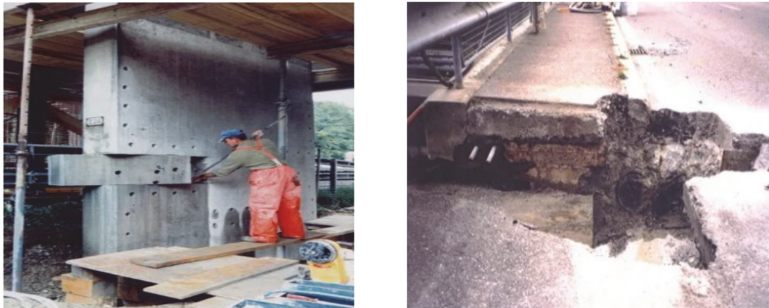
Figure 4: Cutting of pier (left) and failure of anchor heads (right)
