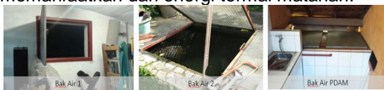
Gambar 8. Instalasi rainwater harvesting
