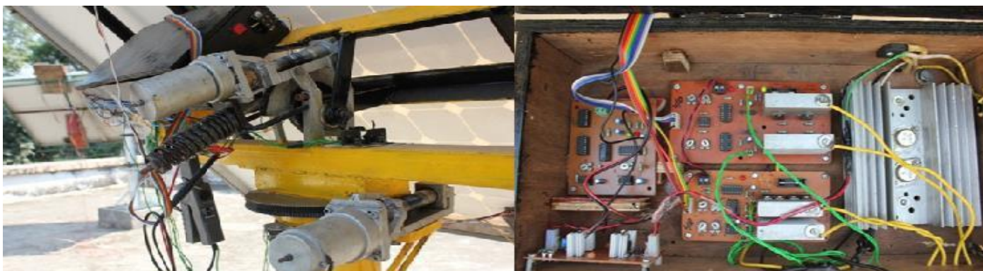
Figure – 1: Electrical Subsystem of Fabricated Solar Tracking System (170X3 Watt)
