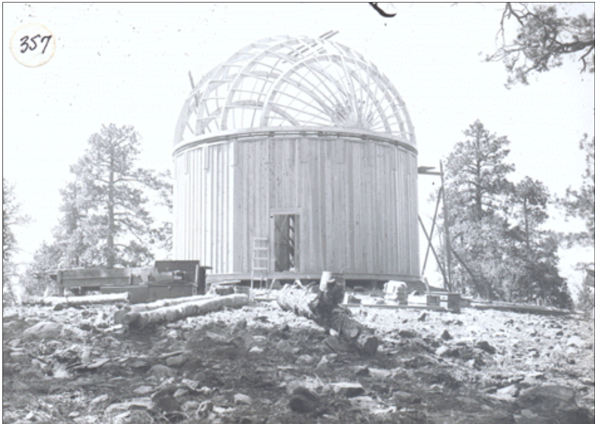
Figure 3: The pre-fab dome designed by William H. Pickering, on Mars Hill, awaiting the arrival of the 18-inch and 12-inch telescopes in May 1894 (courtesy: Lowell Observatory Archives).
