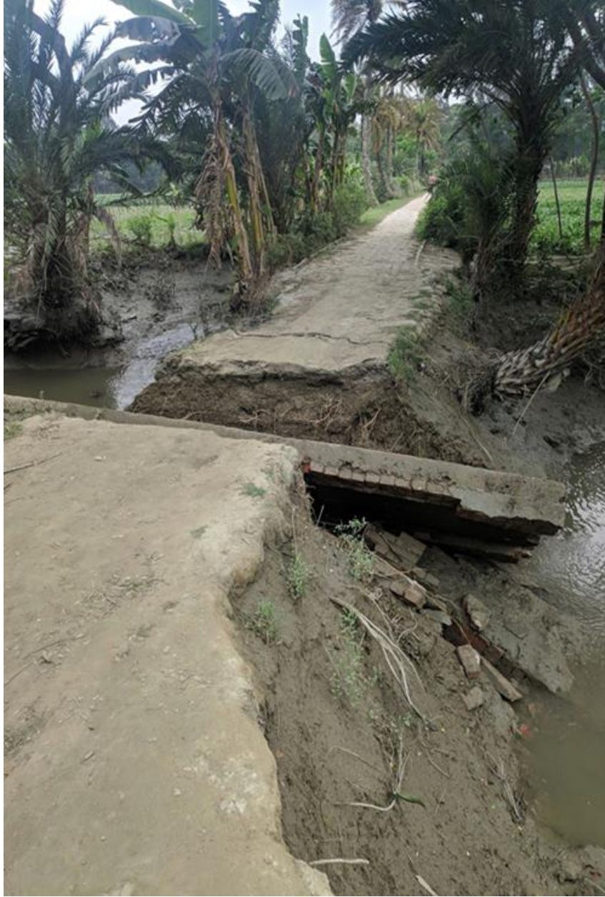
Local culverts are collapsing due to high water velocity in Raghunathpur village, Lakhshampur
