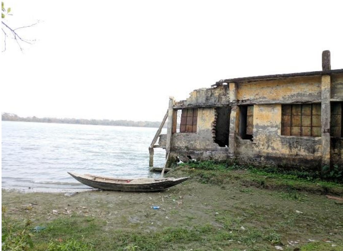
Collapsed school building due to massive erosion of Bishkhali river. Pukhrajana, Rajapur, Jhalokathi
