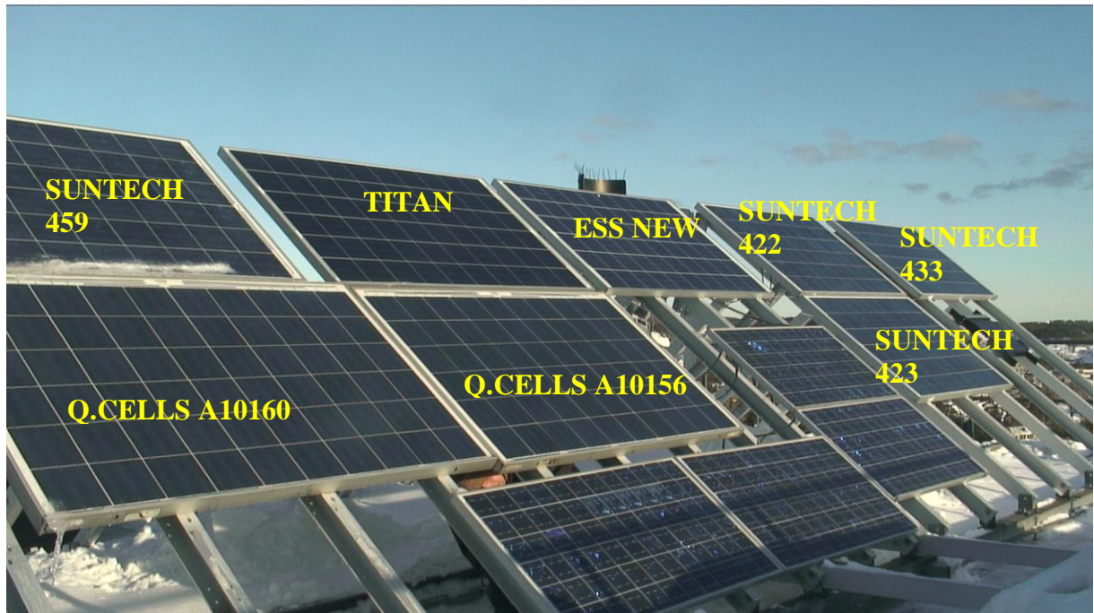
Figure 5.1 – PV research system setup in 2016 located on the rooftop at UiA campus Grimstad. Source: UiA PV Research System.
