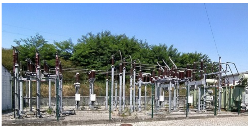
FIGURE 2.1. SE EFACEC Arroiteia (60 kV).
