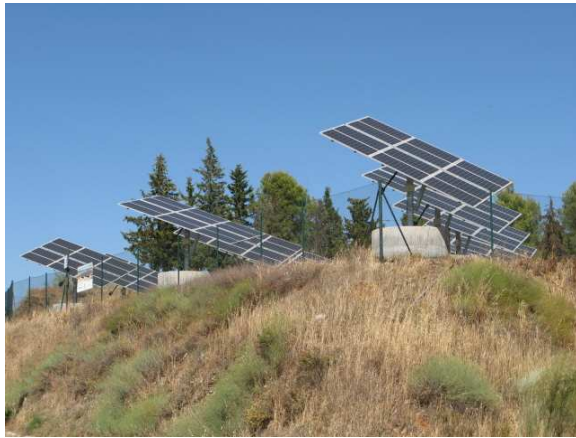
Photovoltaic Panels (Picture: Author)
