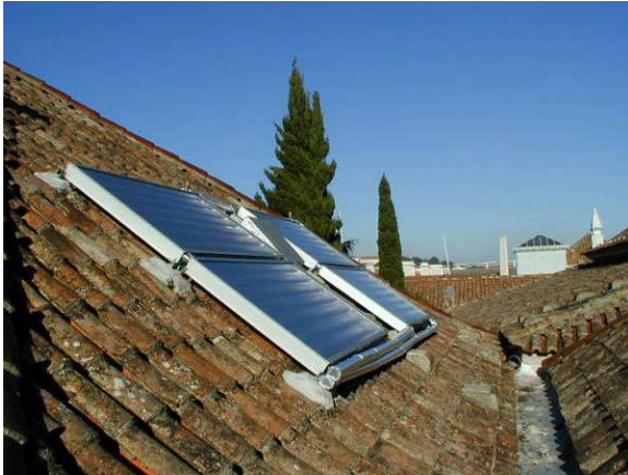
Solar collectors - Lisbon roof (Picture: João F. Saraiva)
