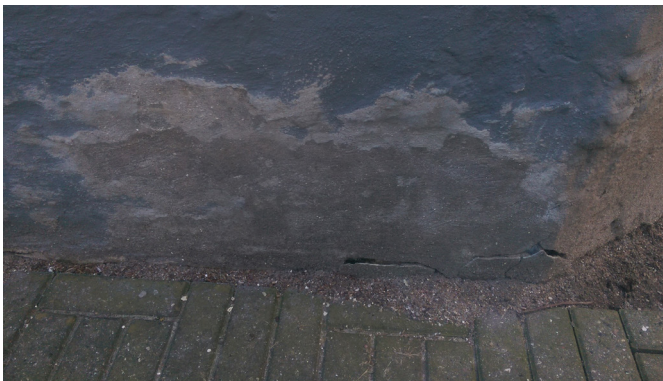
Fig. 21 Facade damage, that was patch up, but the problem persists due to humidity rising from the soil
