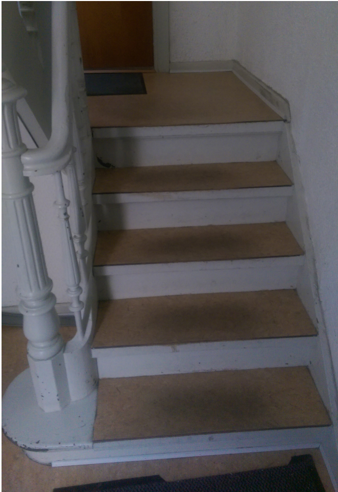
Fig. 27 The main stair case is worn, and should use to be replaced
