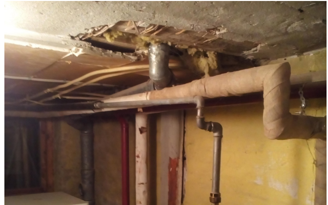
Fig. 20 The pipes in the basement, need to be re-insulated
