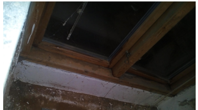
Fig. 26 Basement windows are in really bad shape, and need to be replaced.
