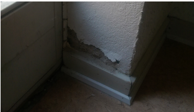
Fig. 25 The paint on the wall in the common access staircase is crumbling.
