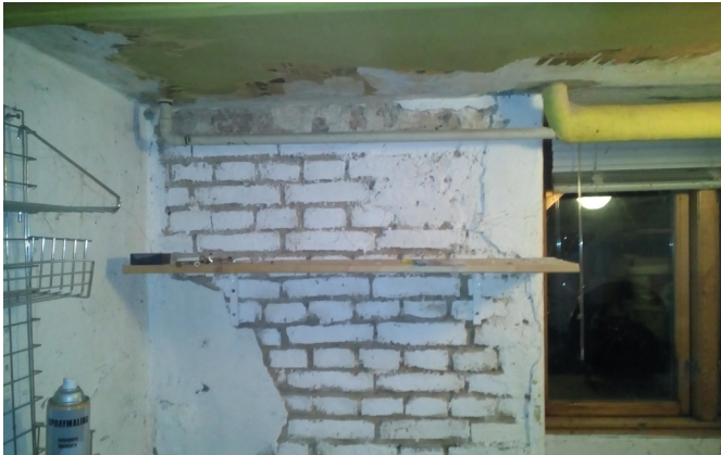
Fig. 19 Basement wall, all in bad state, due to moisture for the soil, most likely the basement doesn't have a damp proof membrane
