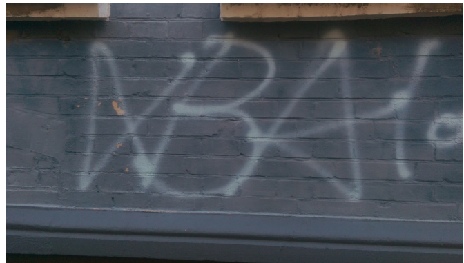
Fig. 22 Vandalism (graffiti) on the facade that need to be cleaned
