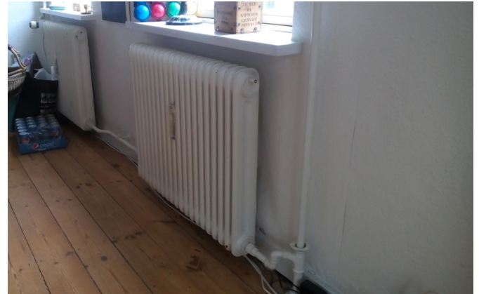
Fig. 24 The radiators are new and are working fine. They will be removed to insulate the building and then put back.
