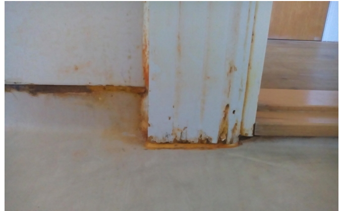
Fig. 28 The bathroom frame door is rooting because of the moisture, the frame has no moisture protection
