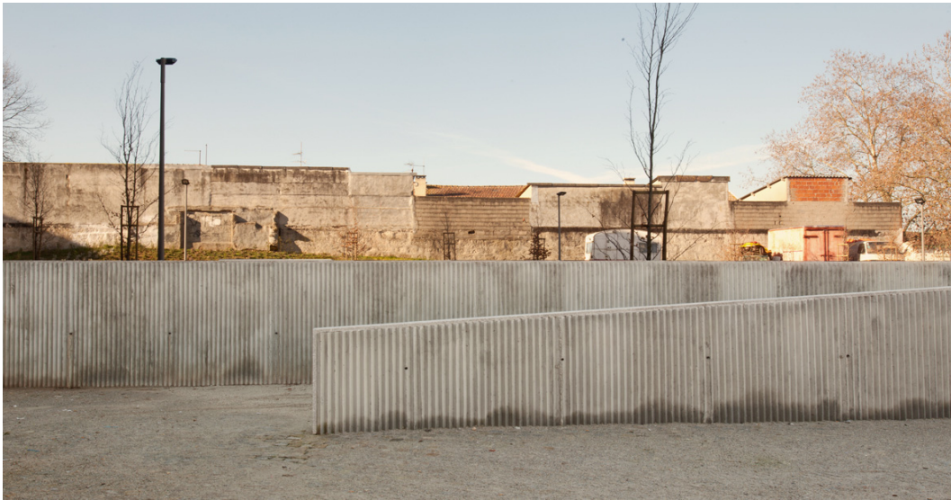
Fig. 6 Detail of the concrete walls, in Lagarteiro, done with special cofferdams (foto by Inês d'Orey).
