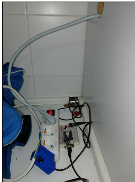
Figure 34 Solution Implementation in the Single Phase Electric Boiler's Source
