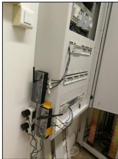
Figure 31 Implementation of the solution in Auditorium C103
