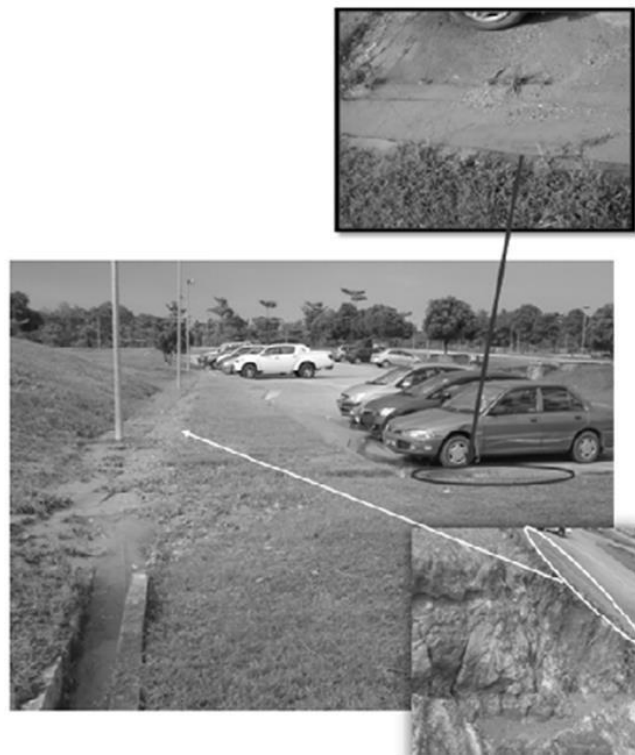
Figure 4: Concrete Drains Choked with Sediments
