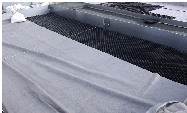
FIGURE 20.9 Installation of a roof barrier sheet in an experimental green roof in Australia. The drainage layer is the black open matrix.
