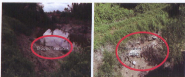
Condition of collapsed bund
