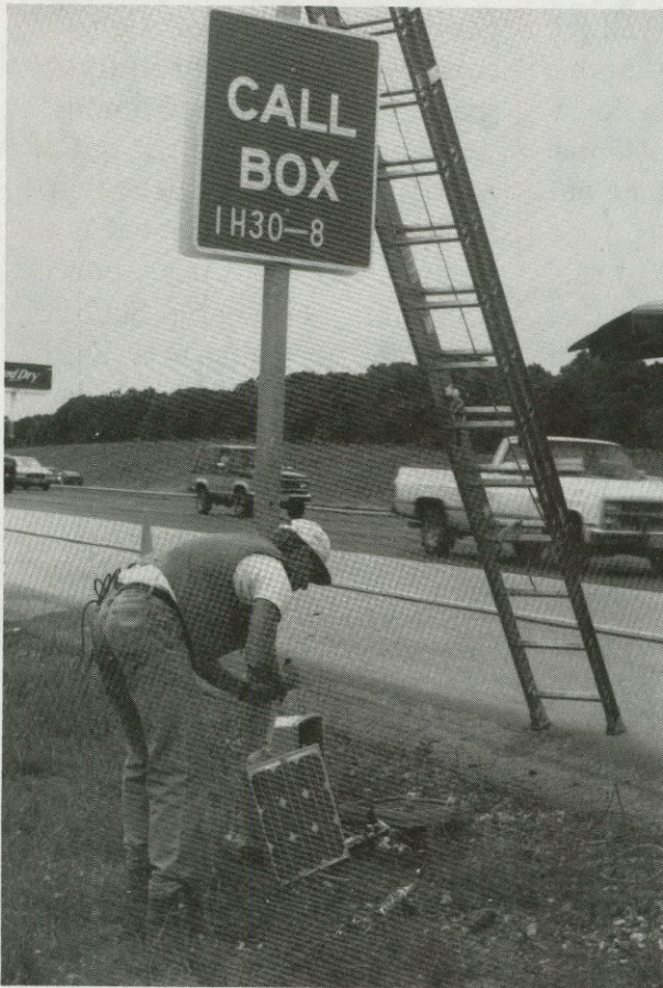
Call boxes—phones along roadways which link callers directly to emergency services—is a joint effort among the 9-1-1 commission, Texas Department of Transportation, and several private companies. Here Larry Buckendahl of GTE Government Information Services prepares to connect the phone to a solar power source. Photo: Steve Barbre
