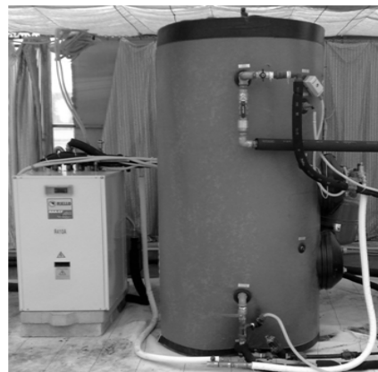
Figure 2. Heat pump and boiler.
