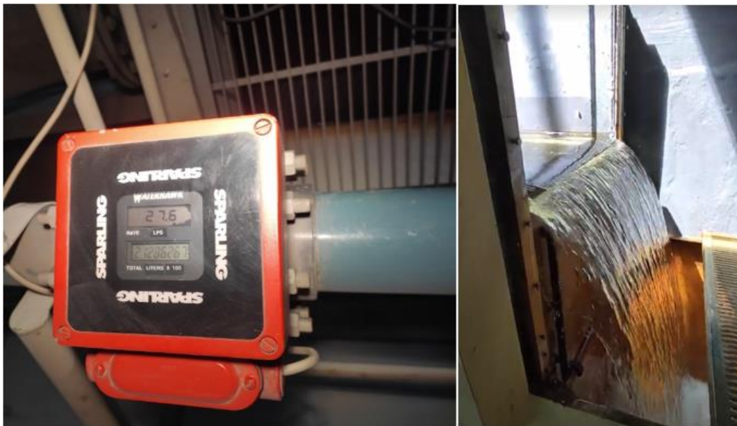
Figure 43 - Flowmeter (Left); Adjustable Mechanical gate (Right).
