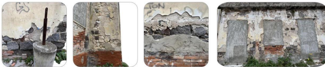
Condition of walls in abandoned building
