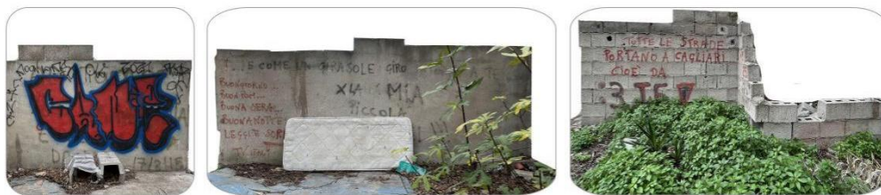
State of the surrounding walls
