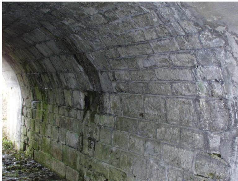
Image 2: Condition of the structure. Wet spots refer to drainage problems
