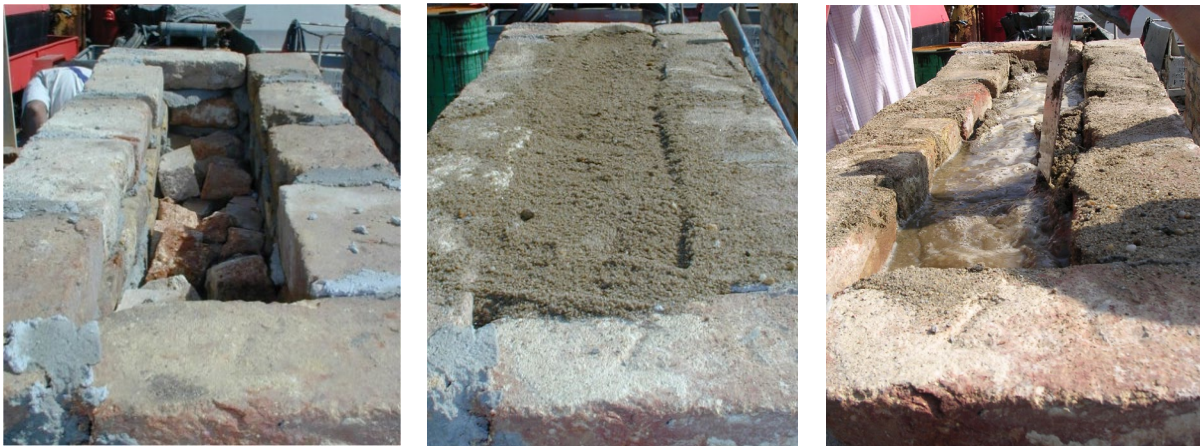
Photo 9. Left: the gap between the courses of F2 wall is filled with debris. Middle: the gap is filled with gravel and sand. Right: the sand in the gap is wetted.
