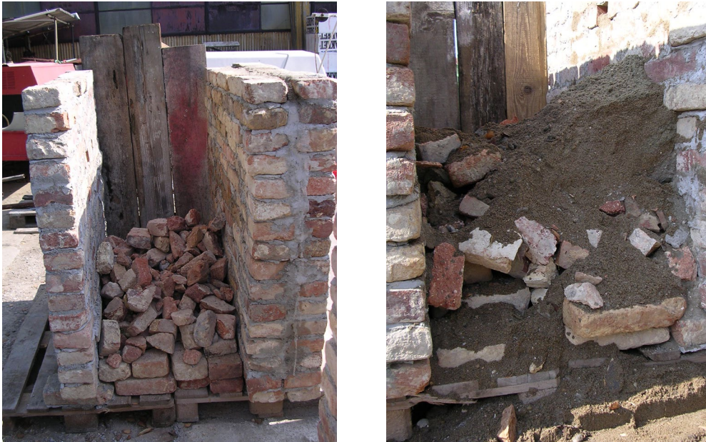
Photo 10. Filling up the gap between F1 and F3 walls with brick debris, gravel and sand
