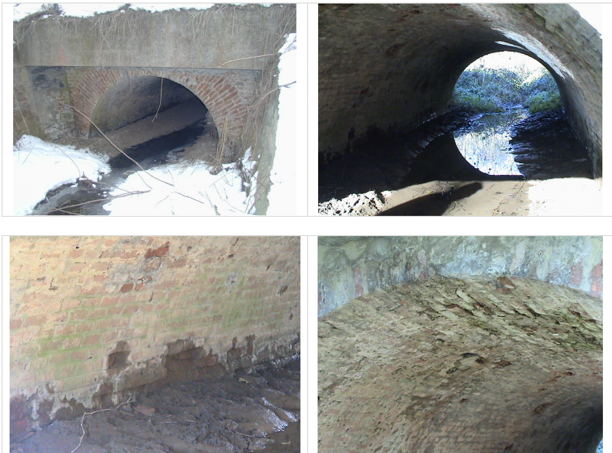
Image 1: Photos demonstrating the condition of the bridge
