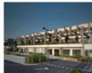
The abandoned concrete skeletons in Carità de Villorba, Italy, to create a multifunctional structure that combined living spaces and common areas into a hotel, a cultural event auditorium and a residence.
