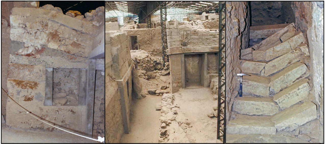
Figure 1. a: Inclination of wall, Sector Delta (from Vougiouklakis 2006: fig. 5); b: Deformation of the upper floors' window sills, Sector Delta (from Vougiouklakis 2006: fig. 4); c: Destruction of staircases, Sector Delta (from Vougiouklakis 2006: fig. 3). Publication rights granted by kind courtesy of the author.
