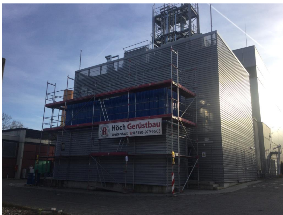
Figure 7: Image of the novel gas treatment plant (background) and the two RWE test rigs (lower container behind cladding: fuel synthesis test rig, upper container: gas treatment test rig).
