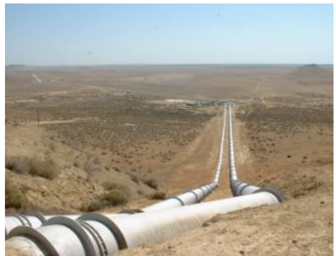
Figure 1. View of the pipeline running from the pump station at the end of the California Aqueduct Coastal Branch up to the Berrenda Mesa Reservoir.
