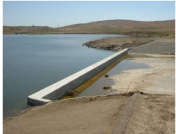
Figure 2. Increased height of bank at the reservoir inlet (top) and increased spillway height (bottom) in Berrenda Mesa Reservoir.
