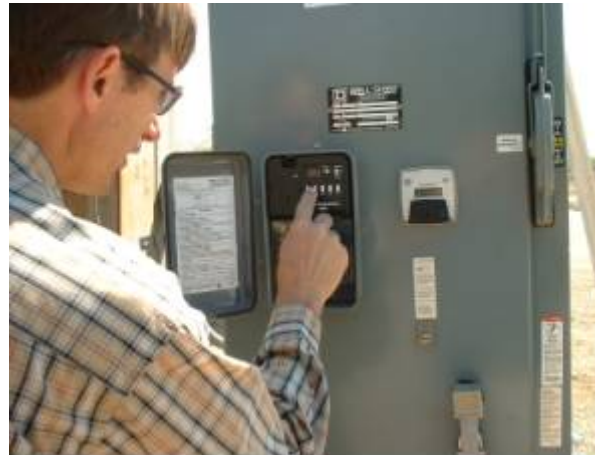
Figure 2. Clock timer used to automatically shut a groundwater well off before 12pm and turn it back on after 6pm every weekday during the peak season.
