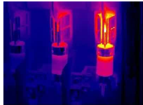
Overheated fuse. Could be caused by a poor connection or the fuse failure. Image courtesy of the Academy of Infrared Thermography.
