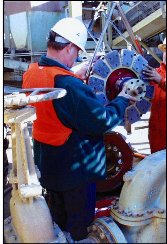
Figure 4. MagnaDrive Installation at Teichert Aggregates. (Photo courtesy of Teichert Aggregates).
