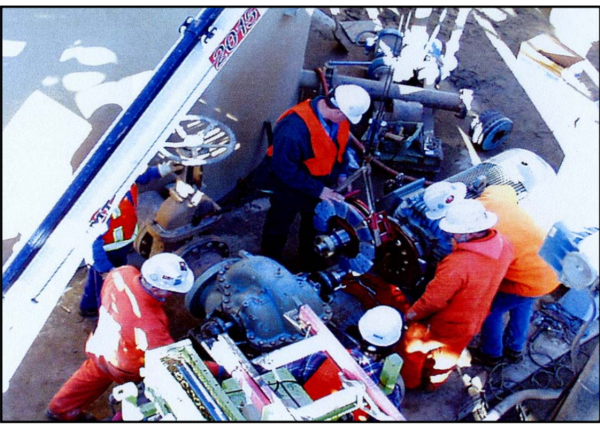
Figure 2. MagnaDrive Installation (Photo courtesy of Teichert Aggregates)
