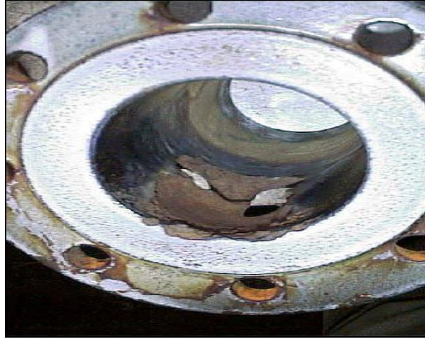
Figure 2-32: Cavitation damage to a gate valve [95].
