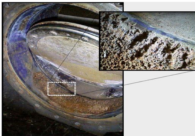
Figure 2-31: Cavitation damage to a butterfly valve [95].
