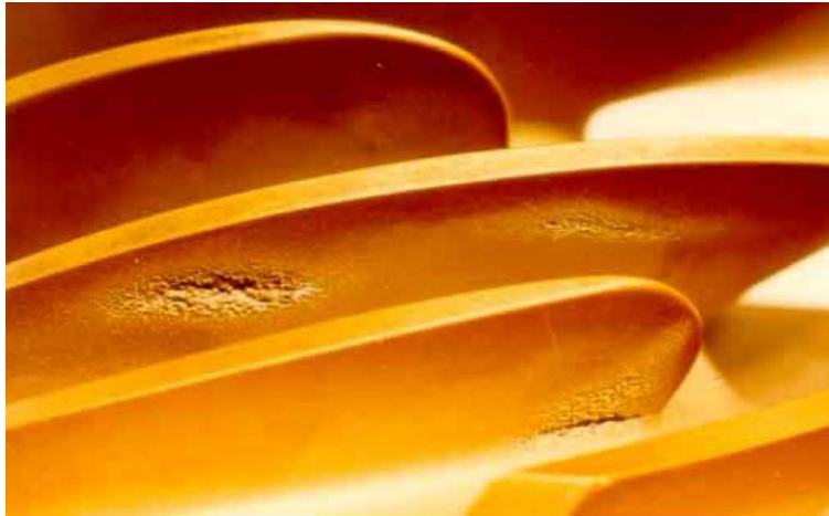
Figure 2-24: Damage caused by cavitation to a closed impeller [6].
